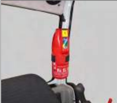
Fig. 88: Fire extinguisher on C pillar
